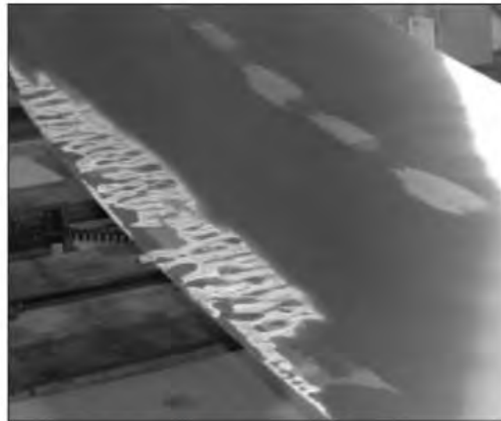
Figure 2 – Water Stain on Sheet
